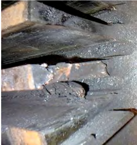
Destroyed rotor forging resulting from undetected ground faults at two locations
